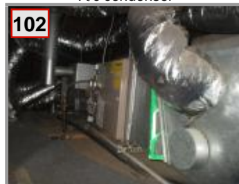
Attic forced air unit.
