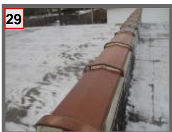
29 Copping stone mortared joints are deteriorated.
