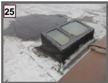
25 Skylights are at the end of there life span.
