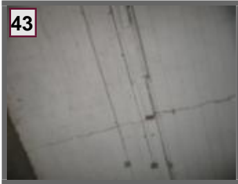
Structure cracks exist.
