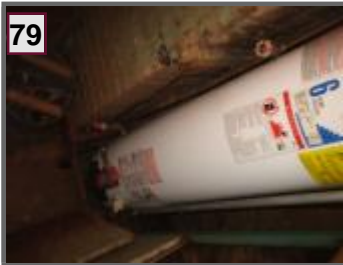
Water heater needs to be replaced.
