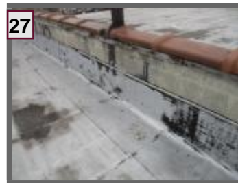
27 Parapet walls need to be weather proofed.
