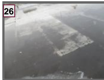
26 Significant amounts of standing water exists on the roof.
