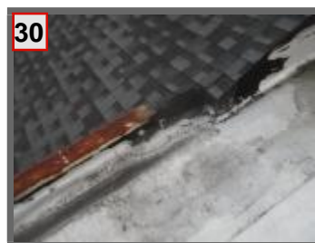
30 Poor repairs have been performed.
